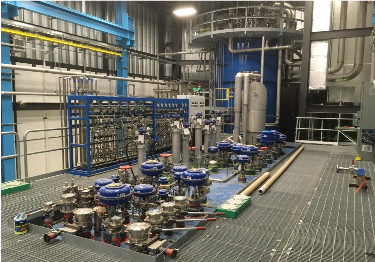
FRIB 4.5 K helium refrigerator cold box (upper and lower sections; cold box room)
