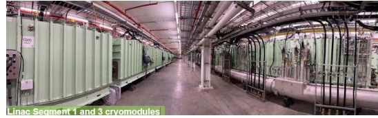
FRIB HWR cryomodules and view of linac (324 resonators in 46 modules all in operation)
